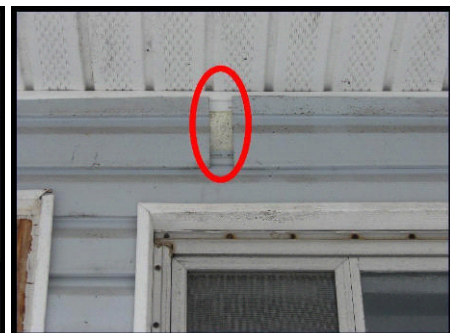
Multiple gaps noted in siding
