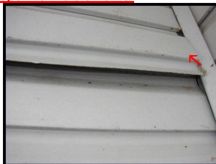
Siding not secured to structure
