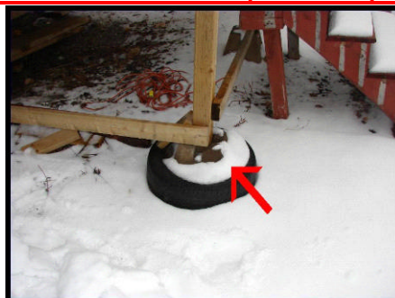
Improper support for deck
