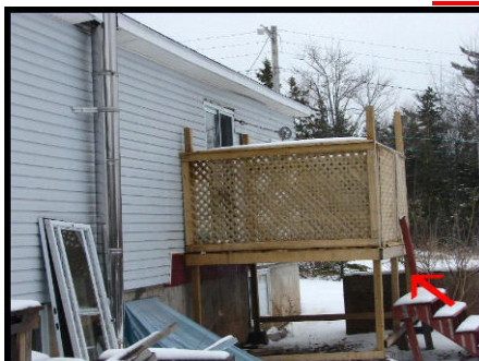
Back Deck. Major issues
